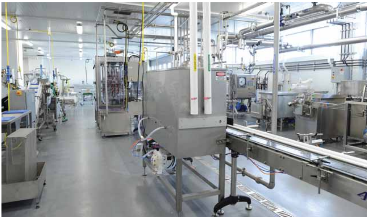
Two of the three food process packaging lines at the IFPT pilot plant include the fresh-vegetable line (left) and the bottling line (center), with clean-up and sanitation equipment strategically positioned nearby on the right to provide students with a real-life food-processing production environment.
